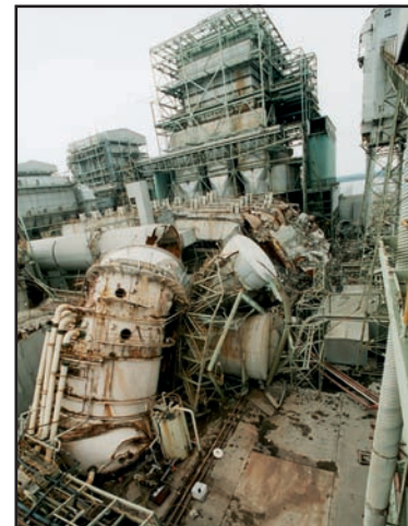
Power plant exhaust stack collapse
