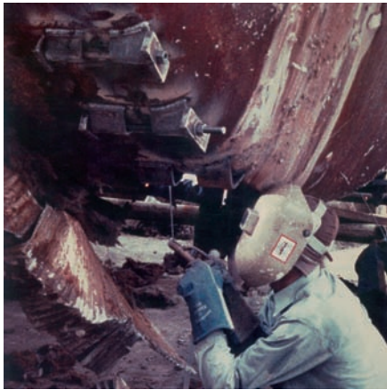
Temporary fix of an essential deaerator tank keeps a paper mill running until the replacement vessel can be delivered
