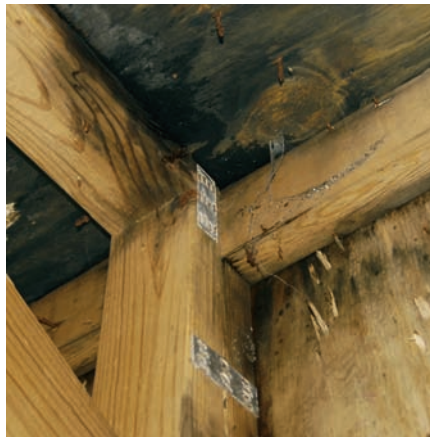
Condensation caused by lack of insulation along exterior wall
